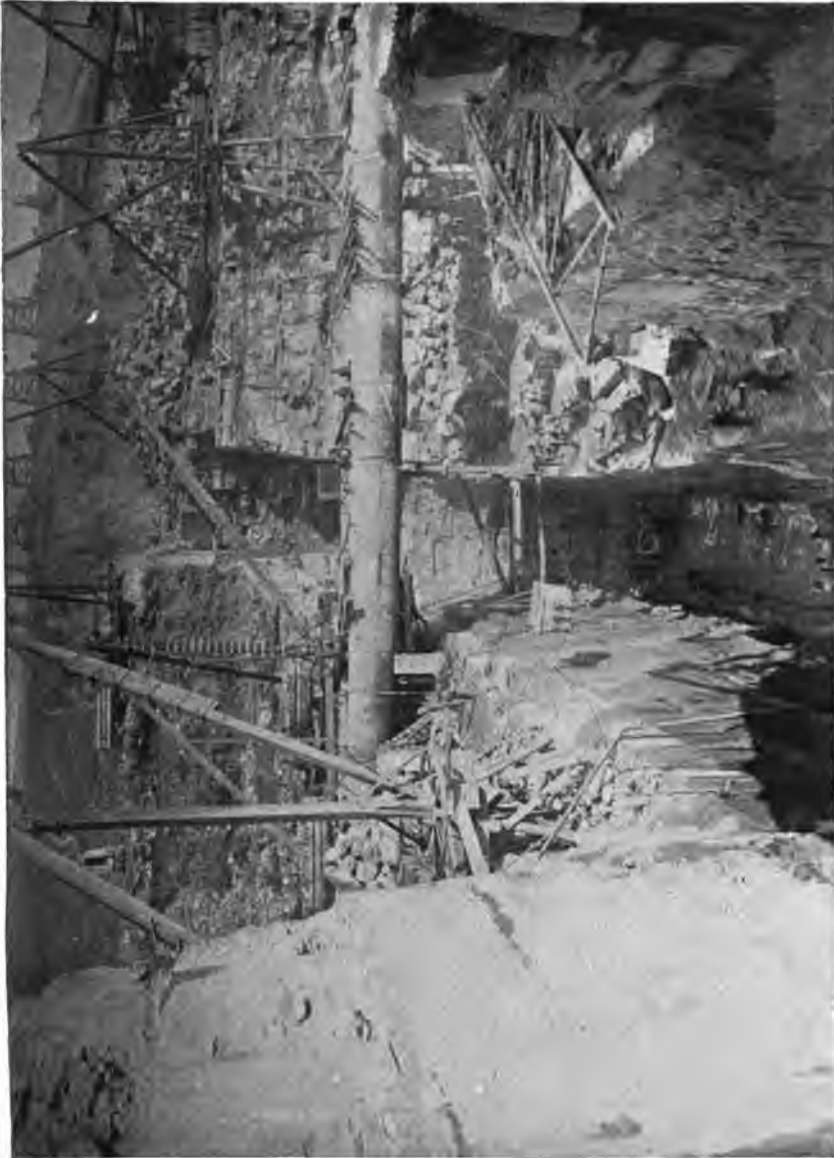
PLATE 35.—View of channelled Cut-off-trench under Upstream Face of Olive Bridge Dam. Two 8-foot Steel Pipes Carrying the Flow of Escopus Creek.
